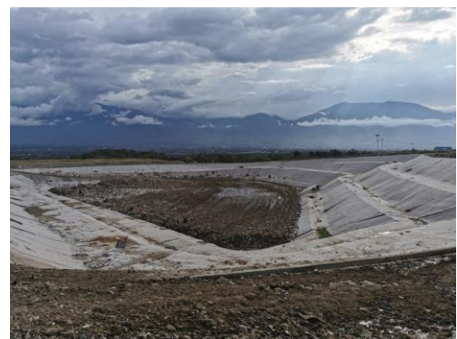
The condition of new cell at Kawatuna Landfill during internal site visit.
